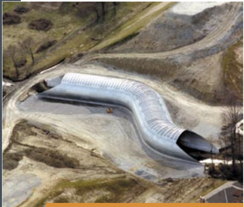
High-profile arch SUPER-SPAN (46'-5" span, 27' rise) in Hamilton, Ohio to span a wetland and to provide a wildlife crossing.
